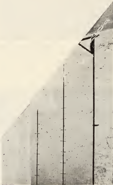
Photo No. 5. A close up of Insulated (metallated) Rocklath Wall (also shown in Photo No. 4) Note Solid Rocklath attached to T-Irons with 16d common nails. Note Horizontal Channel Braces behind T-Irons-which are attached to Anchors in stone wall.
